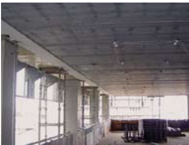
top: The structural frame comprises an optimised mix of insitu and precast concrete elements
