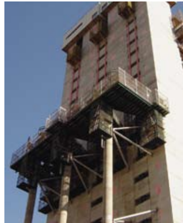
Self climbing 'ClimTrac' formwork was used to construct the three external columns
