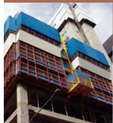
top: Figure 1 Eureka Tower core formwork system showing external stairs with hanging walkways linking all work decks and lobbies to escape stairs (South Side)
