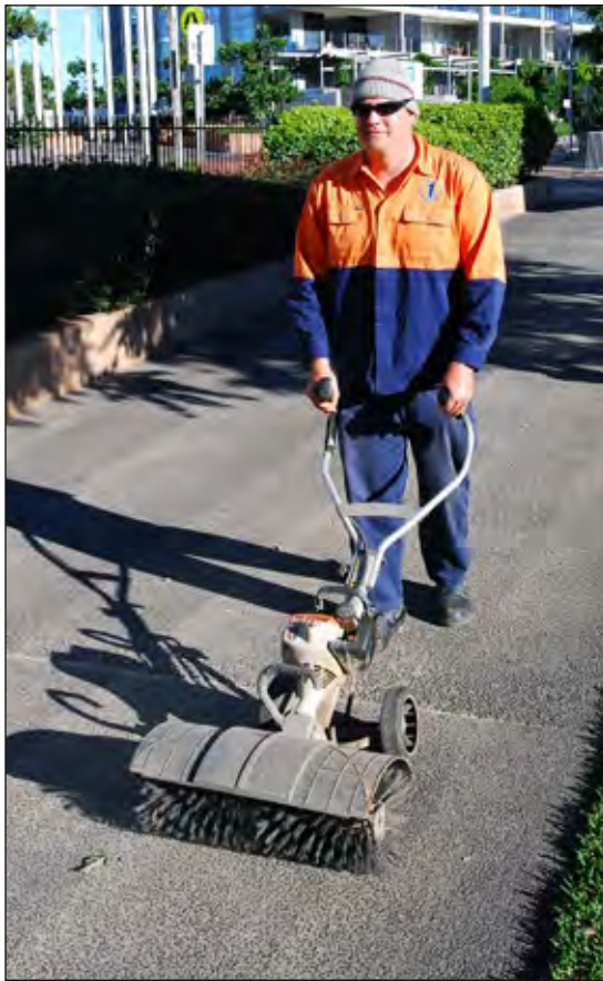
Figure 1: Sweeping a large pavement to remove bulk of loose material prior to pressure washing
